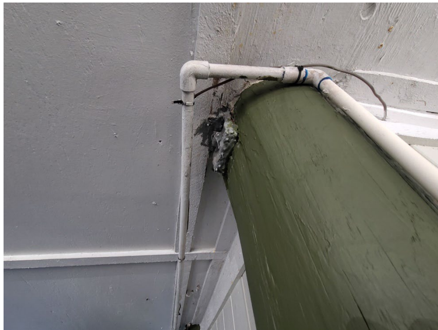
CUSTOM CONNECTION CLIP REQUIRING MAINTENANCE
