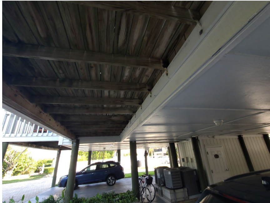
FLOOR JOIST CLIPS REQUIRING REPLACEMENT / MAINTENANCE
