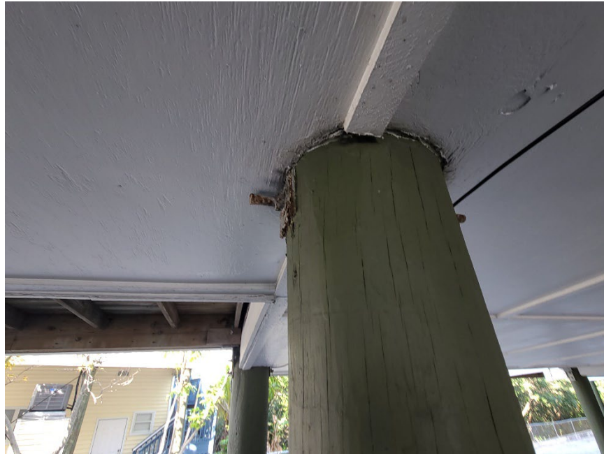
CUSTOM CONNECTION CLIP REQUIRING MAINTENANCE
