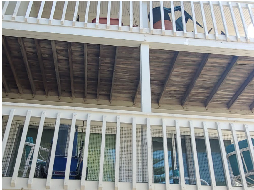
3 RD FLOOR BALCONY FRAMING (PREVIOUS REPAIRS MADE)
